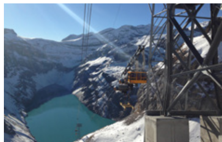
Limmern Pumped Storage Plant, Switzerland
